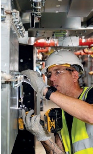
◀ The M&E plant has been relocated to the 'rabbit warren' basement
