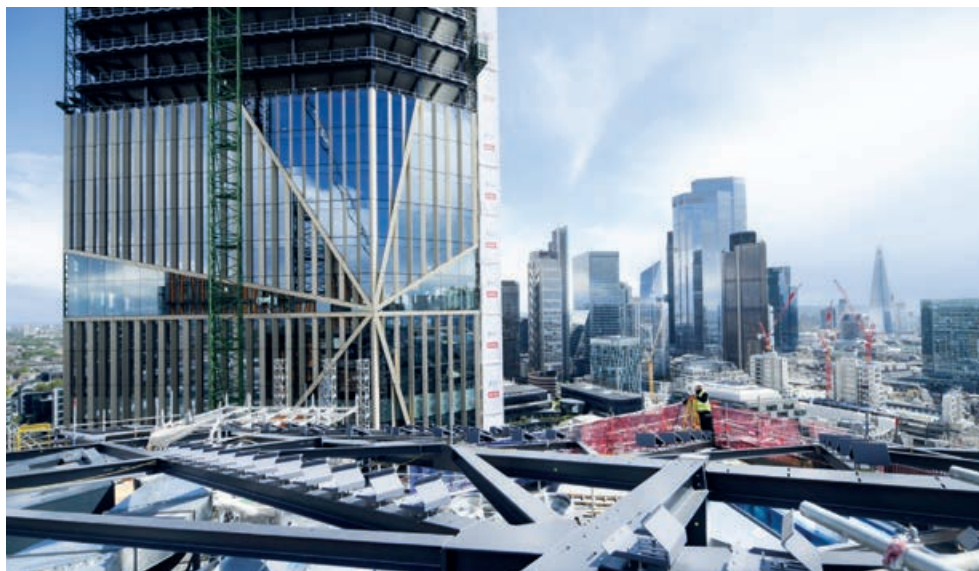
▲ MEP installations on the roof of the west tower, looking towards the taller east tower
