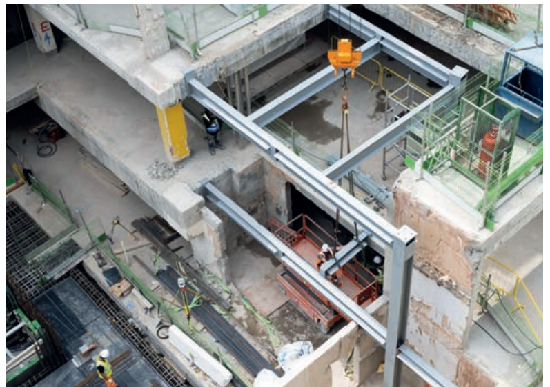
▶ The project reused 16 tonnes of reclaimed steel from the old House of Fraser building
