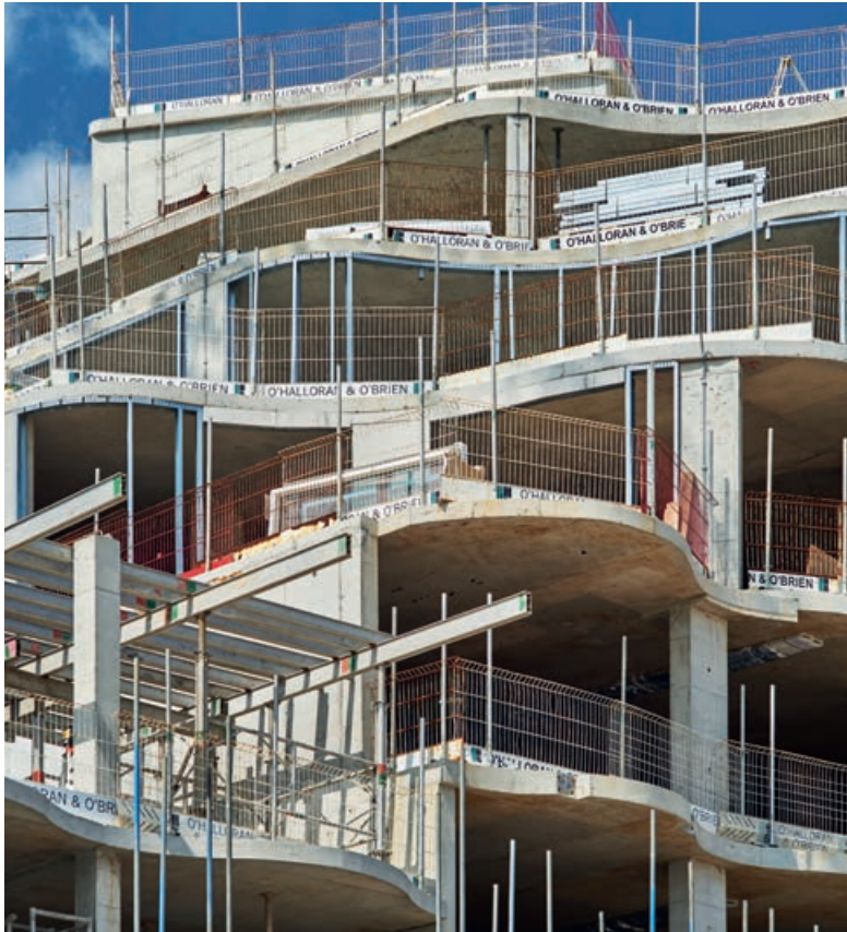
◀ O'Halloran & O'Brien constructed the reinforced concrete frame according to the varying sizes and shapes of the building's curves
