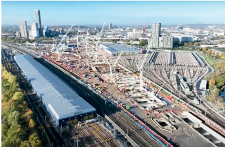
◀ On site at Old Oak Common: "The HS2 station is going to have such a positive impact"
