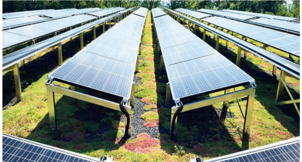
▲ Biosolar roof supplied by Optigreen
