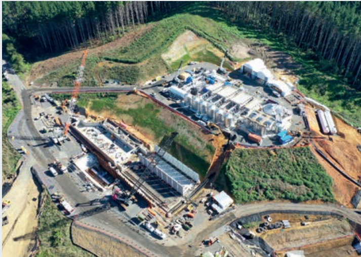
▲ Waikato treatment plant in New Zealand, part of Watercare Services' 10-year, NZ$13bn (£6.16bn) programme of work
