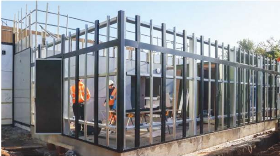
◀ Clockwise from top: the building frame is made from low-carbon steel; a modular unit is craned into place; the wind turbines are erected ▶ Wind turbines supplied by VWT Power offer a source of renewable energy
